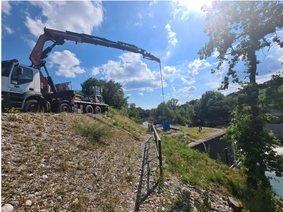
Figure 29: Overhaul of motors and gearboxes, followed by reinstallation at a hydroelectric power plant.
