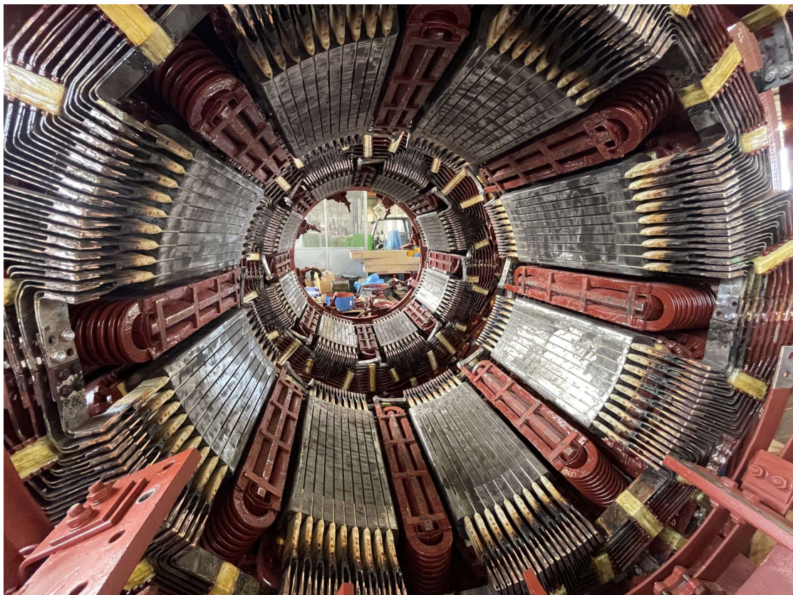
Figure 4: Overhaul and rewinding of a Westinghouse tandem motor of a rolling mill stand, 35.5 kNm.
